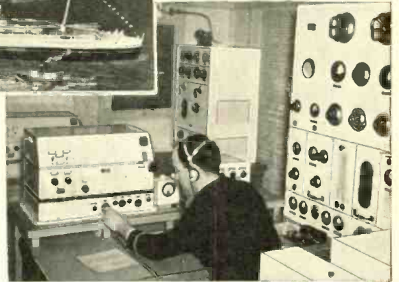
(Photos of radio cabin courtesy A. T. & T. Co., Long-lines Department)
